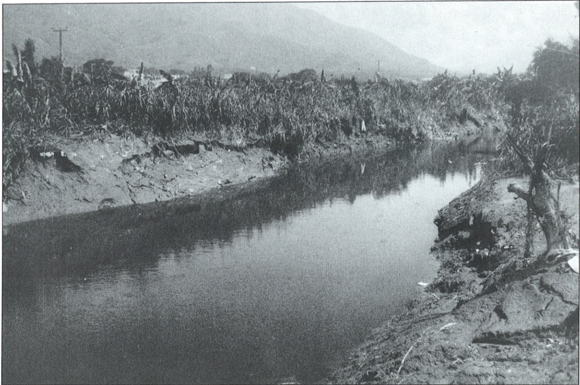
Plate 2a - Bank failure along the Kam Tin River after maintenance works.
