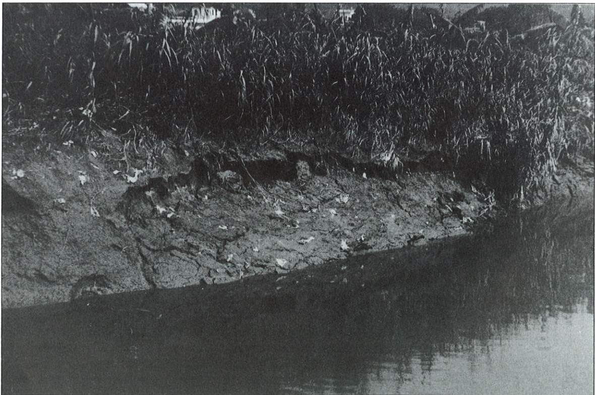
Plate 2b - Bank failure along the Kam Tin River after maintenance works.
